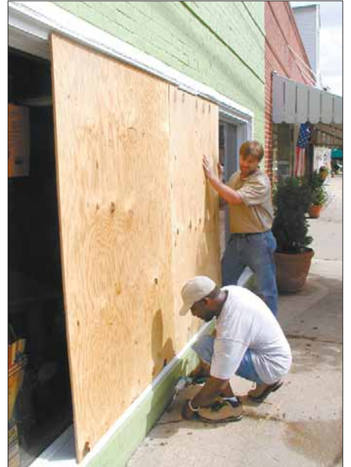
Bill Palmer (left) and Tim Booth of W. F. Booth and Son in Kilmarnock install sheets of plywood to protect the glass storefront on Main Street from the expected wrath of Hurricane Isabel.
